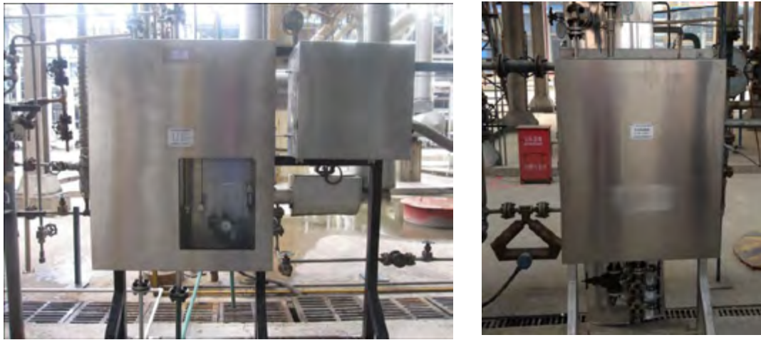
Figure 4. On-site sampling cabinet of Analysis system
