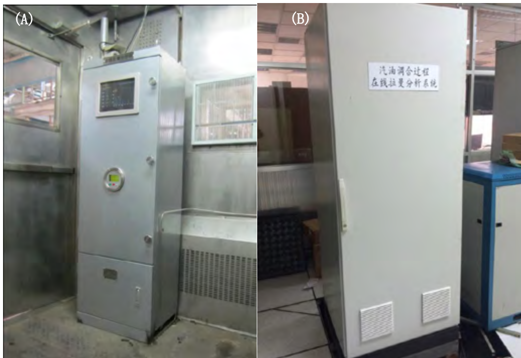
Figure 5. Main cabinet of analysis system:
