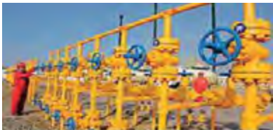
Natural gas pipeline valves
