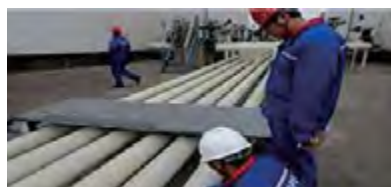
Oil and gas transmission pipeline
