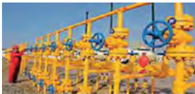
Natural gas pipeline valves
