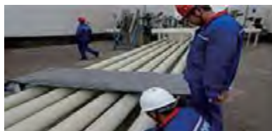
Oil and gas transmission pipeline
